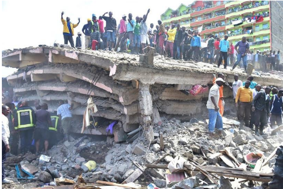
Collapsing of buildings
